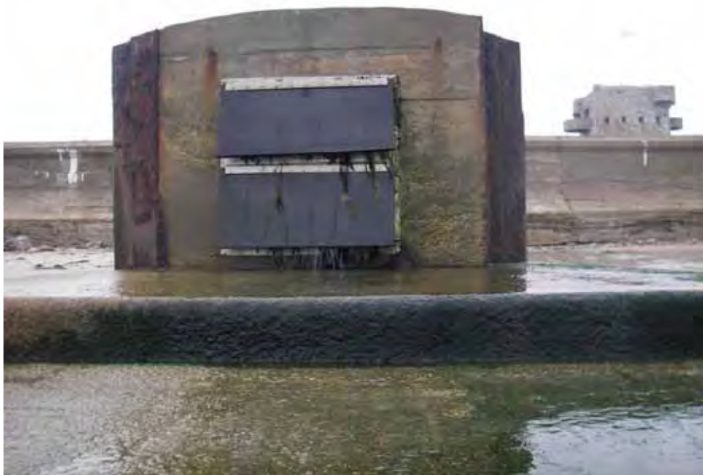
Figure 14. Outfall with double flap valve near Fort Henry
