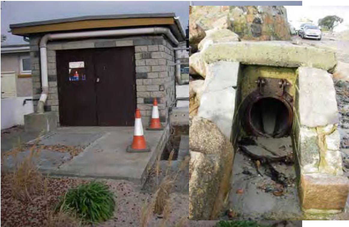
Figure 4. Pumping Station and associated discharge pipe at Le Hocq
