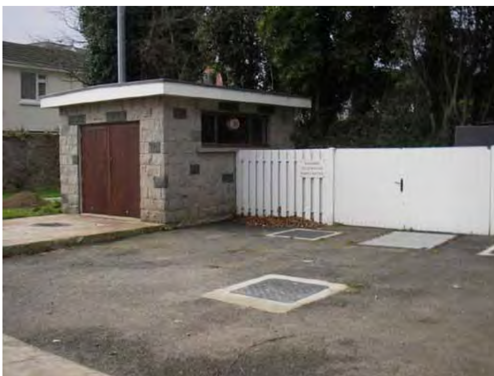
Figure 9. Pontac Pumping Station
