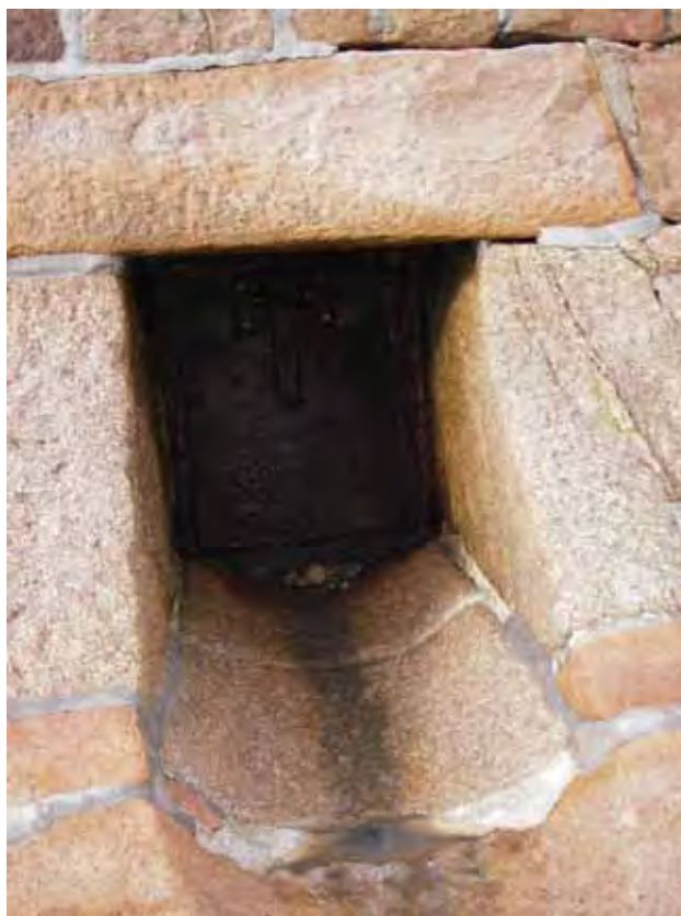
Figure 10. Flap valve in sea wall at Le Hocq
