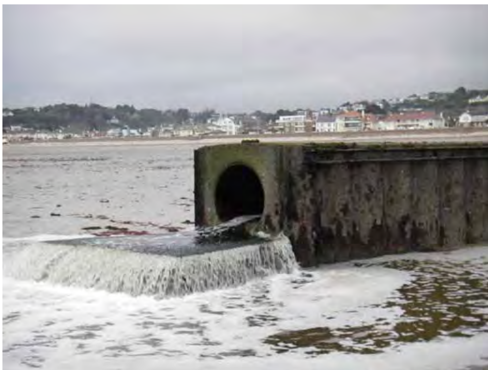
Figure 11. Main Bellozane outfall
